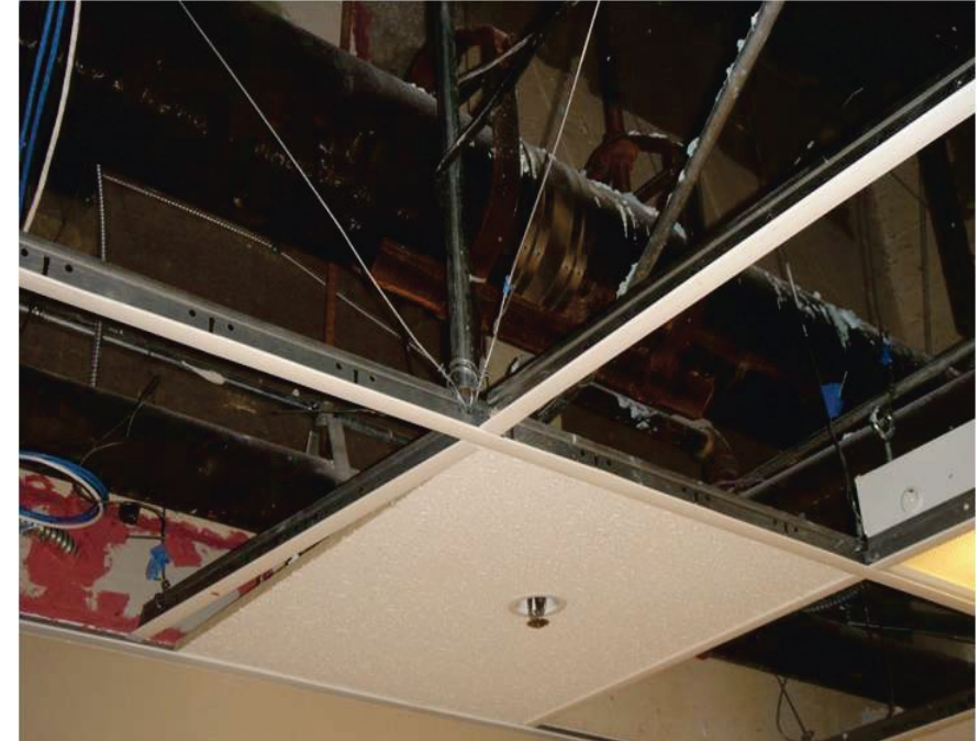
Suspended Acoustic Tile Ceilings Restrained by Compression Struts and Diagonal Splayed Wires (from FEMA E-74, 2012, Reducing the Risks of Nonstructural Earthquake Damage—A Practical Guide )
