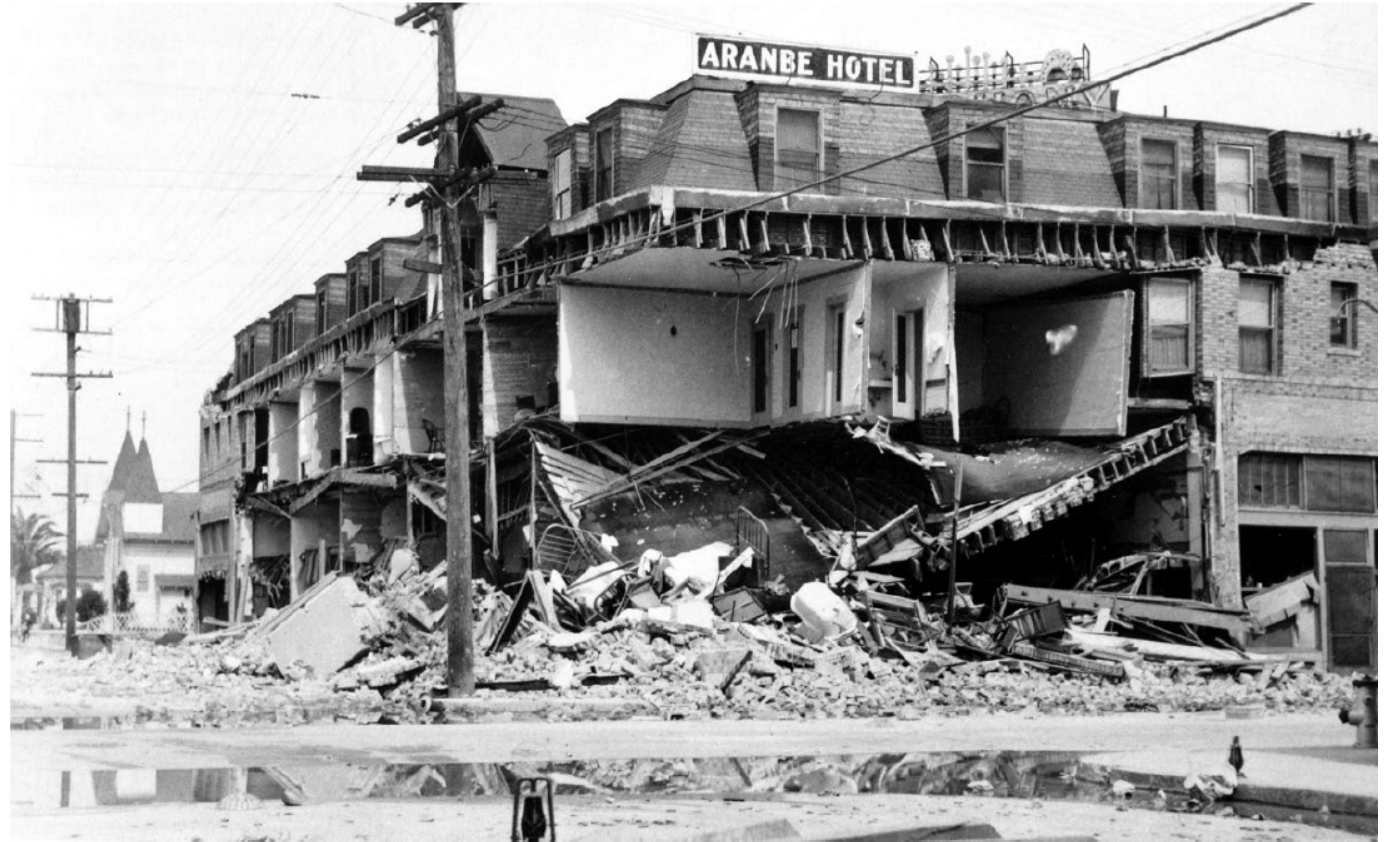
URM Bearing Wall Damage in the 1933 Long Beach EQ (from FEMA P-2156 and Los Angeles County Library)
