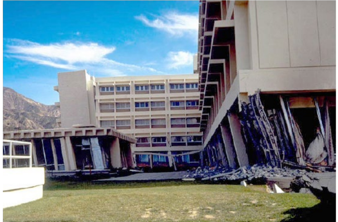
Excessive Drift at the Soft Ground Story of the Olive View Hospital in the 1971 San Fernando EQ (from FEMA P-2156 and William Godden, NISEE-PEER)
