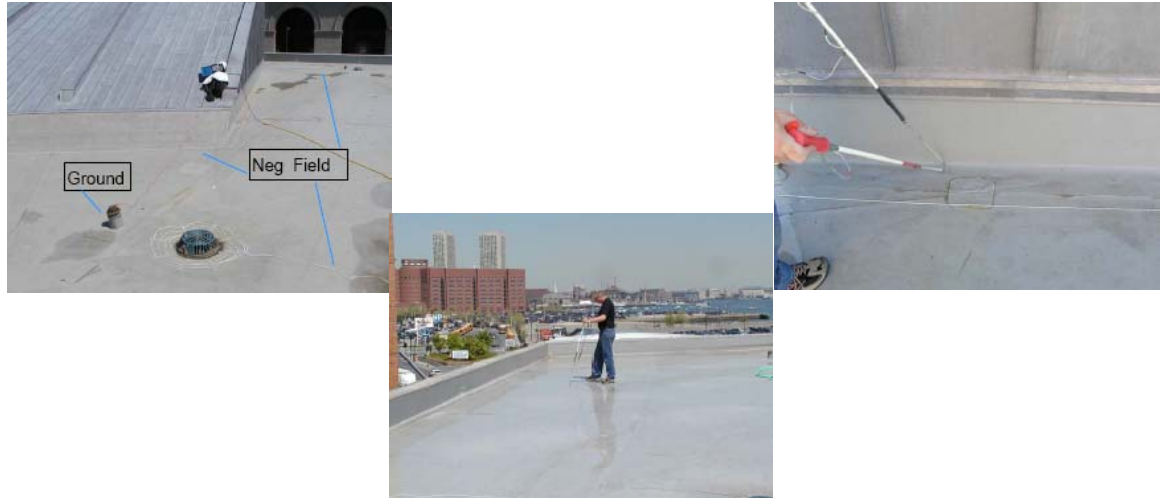
Figures 15 through 17 for roofing, waterproofing and vegetated roofs, Electric Field Vector Mapping is an extremely useful and accurate tool for pin-pointing leaks.
